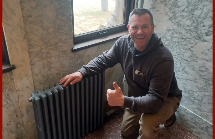
New radiators and pipes were installed, saving Director of Facilities and Grounds Marc Stanek countless hours each winter morning.
